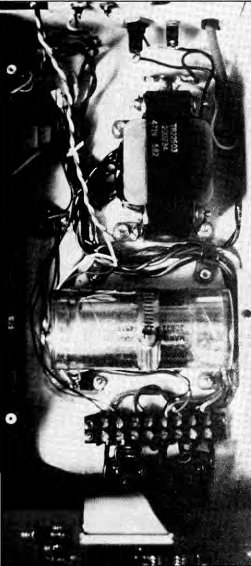
Photo 1. The power supply of the LNW-80 is quite hefty. I have used heavy-duty bridge rectifiers bolted to the case (partly shadowed, bottom right) and fed through barrier strips. An automotive cable clamp holds a large filter capacitor, and all the wires are hanked together with plastic clamps and bolted to the case. A power supply is created for an integral disk drive using the added heft of the LNW-80 transformer; 5- and 12-volt regulators are visible just above and below the left side of the filter capacitor.
