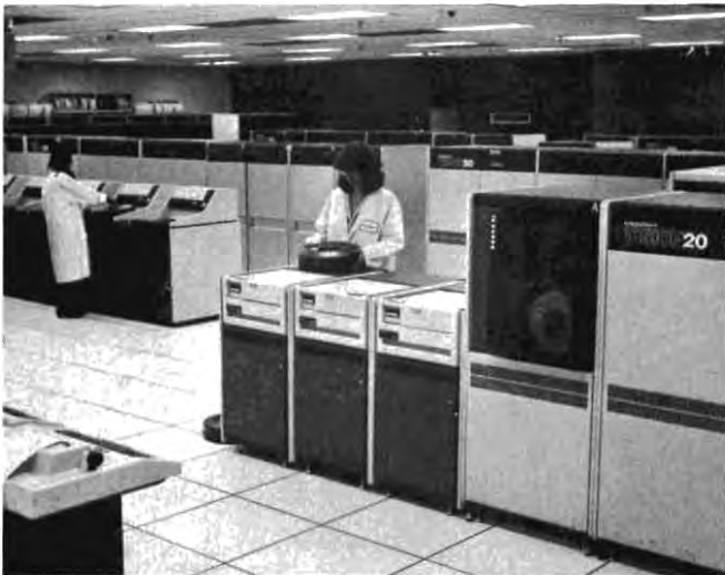
Of CompuServe's 22 large computer systems, 10 are housed here in our Dublin, Ohio Computer Center.
